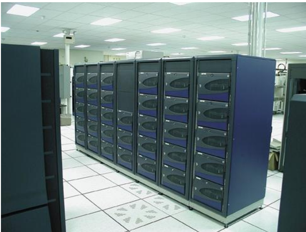
Figure 1. The Cluster as Finally Installed
